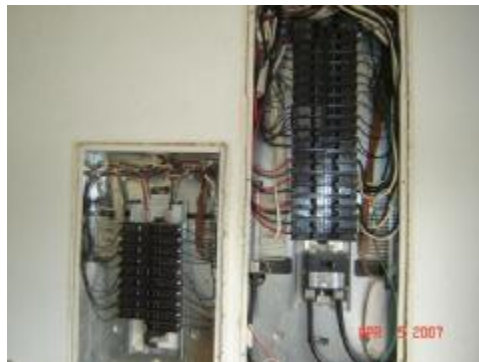
Main and auxiliary distribution panels.
